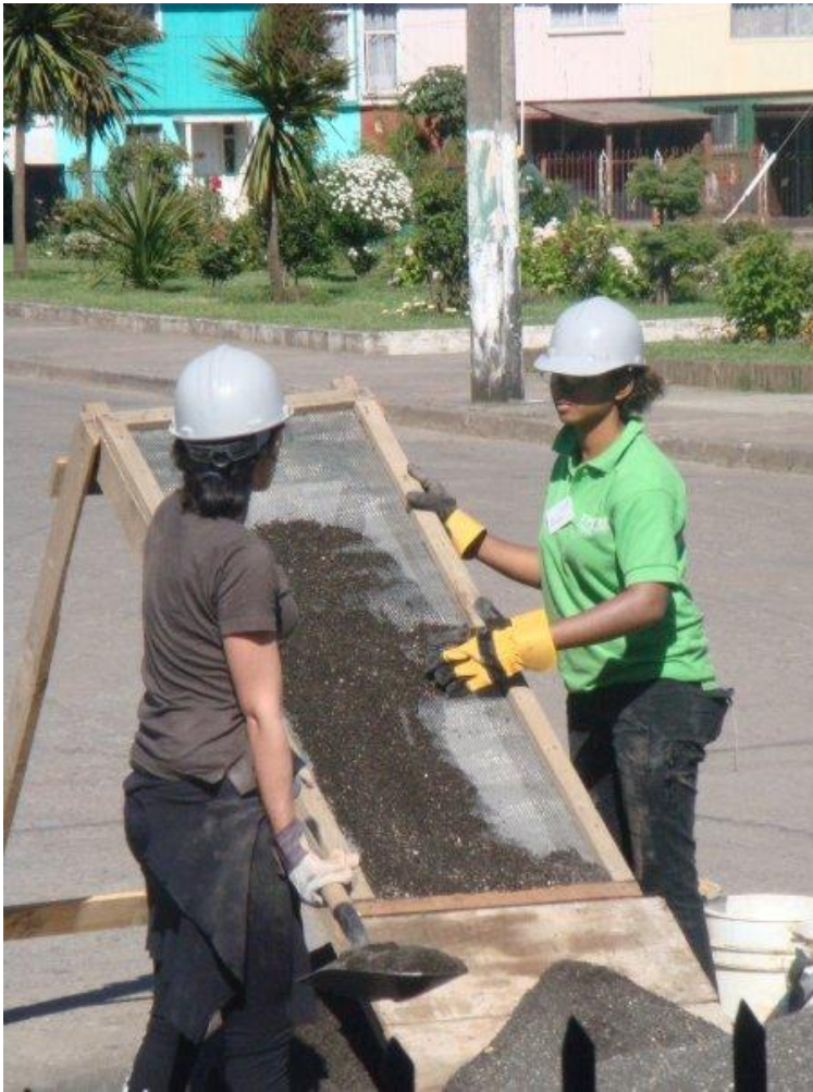
Alexandria and I sifting the sand so that mortar can be made
